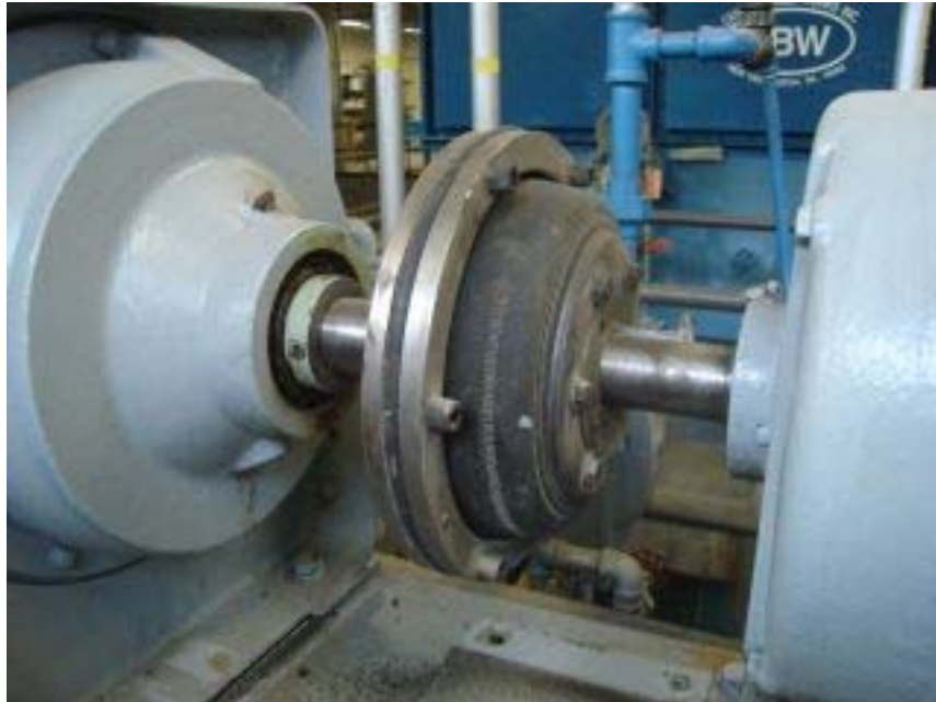
Figure 18a old boiler coupling
