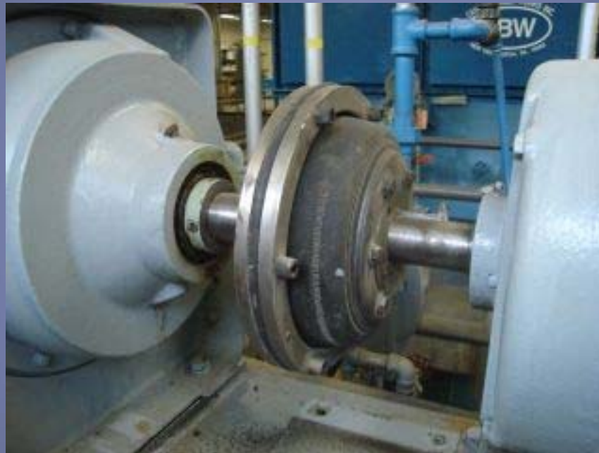
Old boiler coupling
